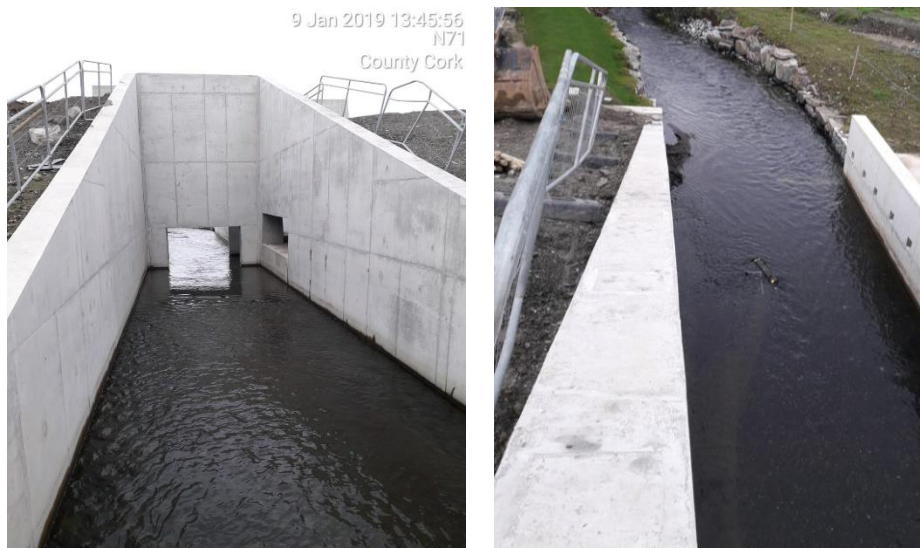
Water flowing through the flow control structure
